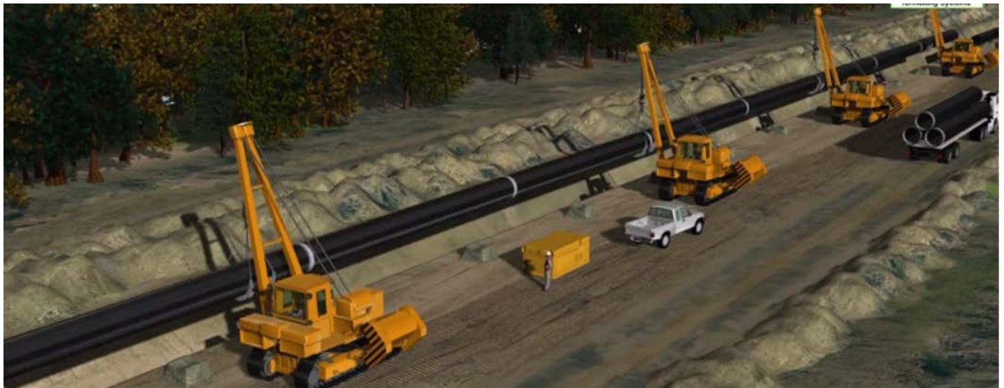
Conventional method: Pipe laying cranes place pipe in open cut excavation, which will then be backfilled
