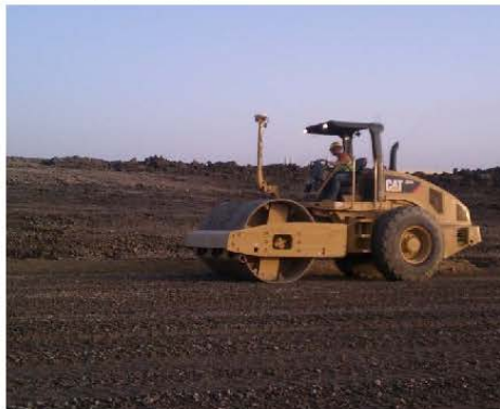
Shown is NorthGate equipment utilizing the intelligent compaction software, with the receiver at the top.
