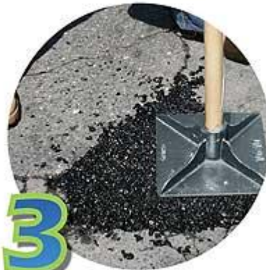
3 Add GreenPatch up to a 2" depth and compact to create a solid base. Reapply in 2" increments until repair area is filled. Leave a small "crown" to allow for further compaction. You may open to traffic immediately.
