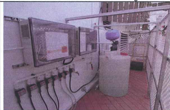
Chillers Water Reuse for Harvesting – for irrigation purpose.
