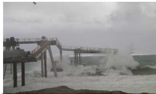
Catwalk used to interconnect structures
