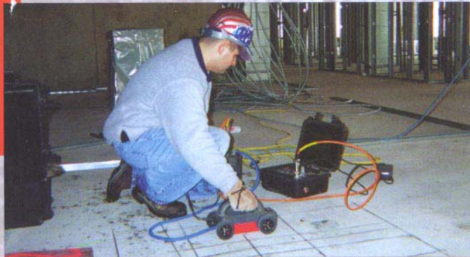
While scanning the area where a penetration is needed, the operator marks the locations of the post tensioned cables.
