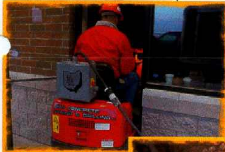
Operator driving unit through a 32" doorway. Note, electric cord instead of diesel exhaust.
