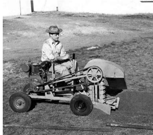
The DWP trencher is used to prepare for the installation of a water line.
