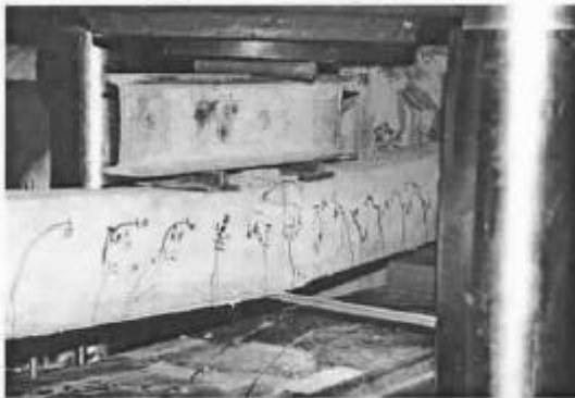
Beam reinforced with carbon FRP tested to failure
