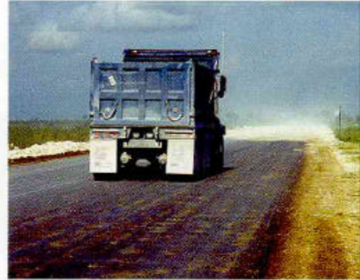
This is an unpaved quarry road located in Coral Springs, Florida, stabilized with RB Ultra Plus™. The average trip count is 200+ trucks per day, with loaded weights of 60,000 to 80,000 lbs. Before using RB Ultra Plus™ the road needed to be watered 2 to 3 times a day for dust control and graded to keep the road open. After using RB Ultra Plus™ watering was reduced to once every 6 weeks and grading was reduced to once a month.
