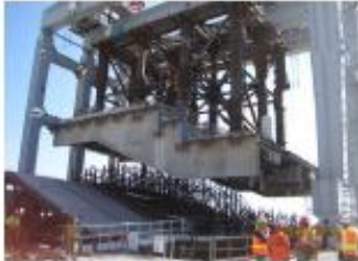
Super Gantry Crane—largest of its kind—capable of lifting up to 5,300 tons.
