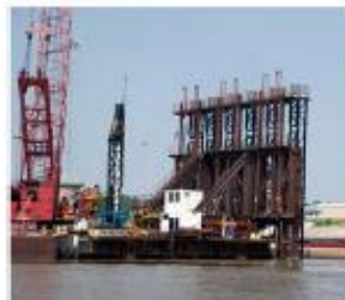
This innovation saved valuable budget dollars and eliminated many diving and salvaging operations which improved project safety.
