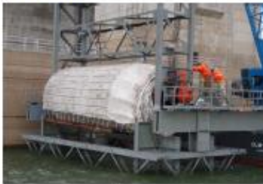
Grout mat being lowered through the guide frame to the river bottom.
