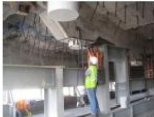
URS developed a first-of-its-kind air pressure system installed beneath the concrete shell.
